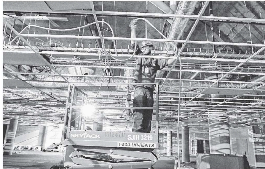
Wade Grisenthwaite, from Dayton, Pa., takes down lighting in Eastman Business Park Building 326 on Tuesday. Kodak will partner with UniPixel Displays Inc. of Texas to manufacture touch screen sensors at the Greece location. SHAWN DOWD/STAFF PHOTOGRAPHER
